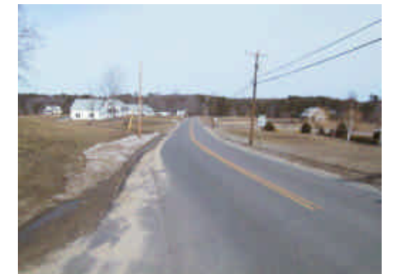
State Road/Rt 103, Eliot, needs shoulders
