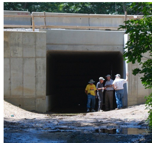
A glimpse into the future — the culvert under Route 109 in Wells, Maine
