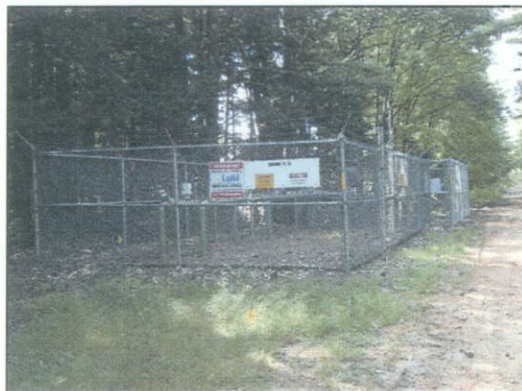
E13: Unitil regulator station near Cascade Road crossing
