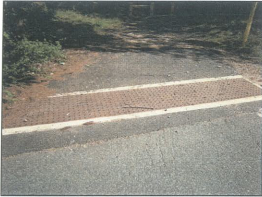
Example of cast iron detectable warning plates used on Scarborough trail section.
