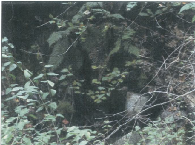
Outlet looking northwest
