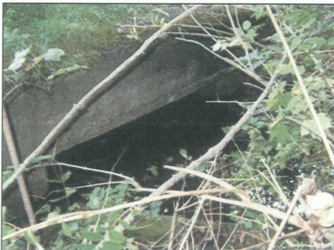
Outlet looking northwest
