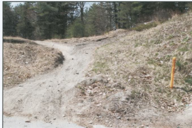
South view of eastern side of abutment; may not fall on ETMD property
