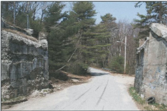
West View – Paths on west side of abutments obstructed
